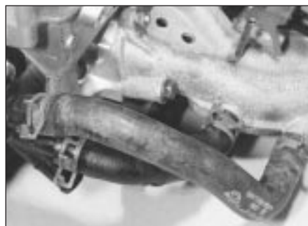
11.5 Coolant hoses in position
