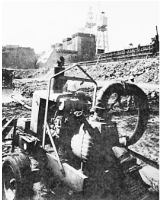
Figure 9-7 Self-priming centrifugal pump at dam construction site. (Courtesy of Crane Pumps & Systems)
