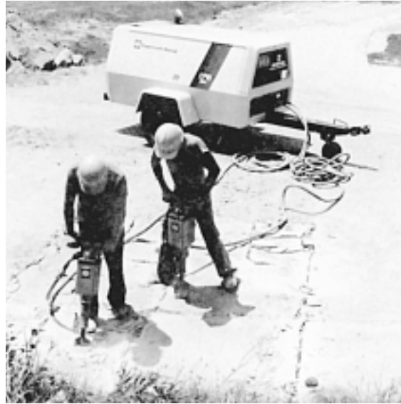
Figure 9-2 Small portable air compressor powering pneumatic tools. (Courtesy of Ingersoll-Rand Company)
