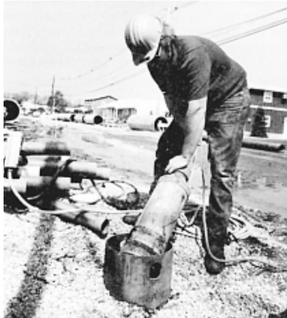
Figure 10-23 Electrically powered submersible pump being placed into dewatering well. (Courtesy of Crane Pumps and Systems)
