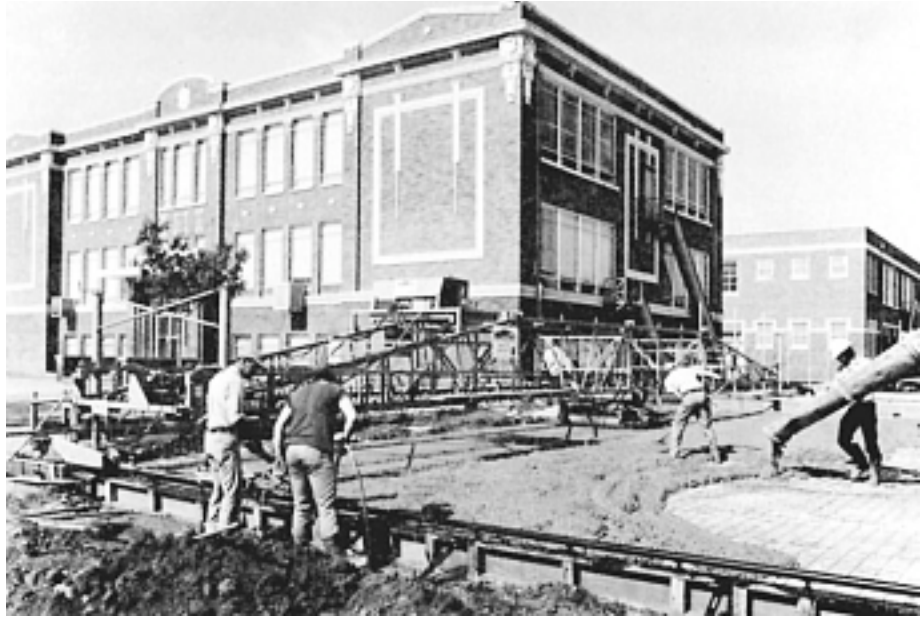
Figure 12-17 Roller finisher being used on large slab pour. (Courtesy of Terex Roadbuilding)
