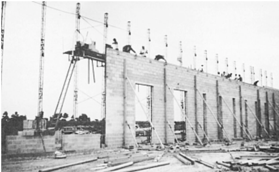
Figure 14-24 Bracing of a concrete masonry wall under construction. (Courtesy of Portland Cement Association)
