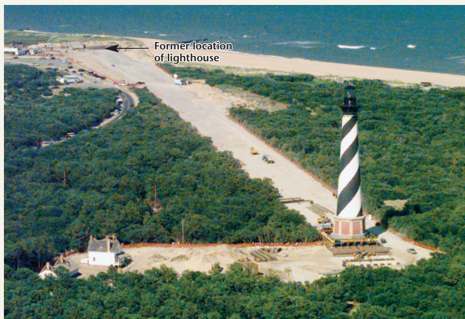
FIGURE 20.B Cape Hatteras Lighthouse after being moved 488 meters (1600 feet) from the shoreline. At its new location it should be safe for 50 years or more. (Photo by Reuters/Stringer/Getty Images, Inc.—Hulton Archive Photos)
