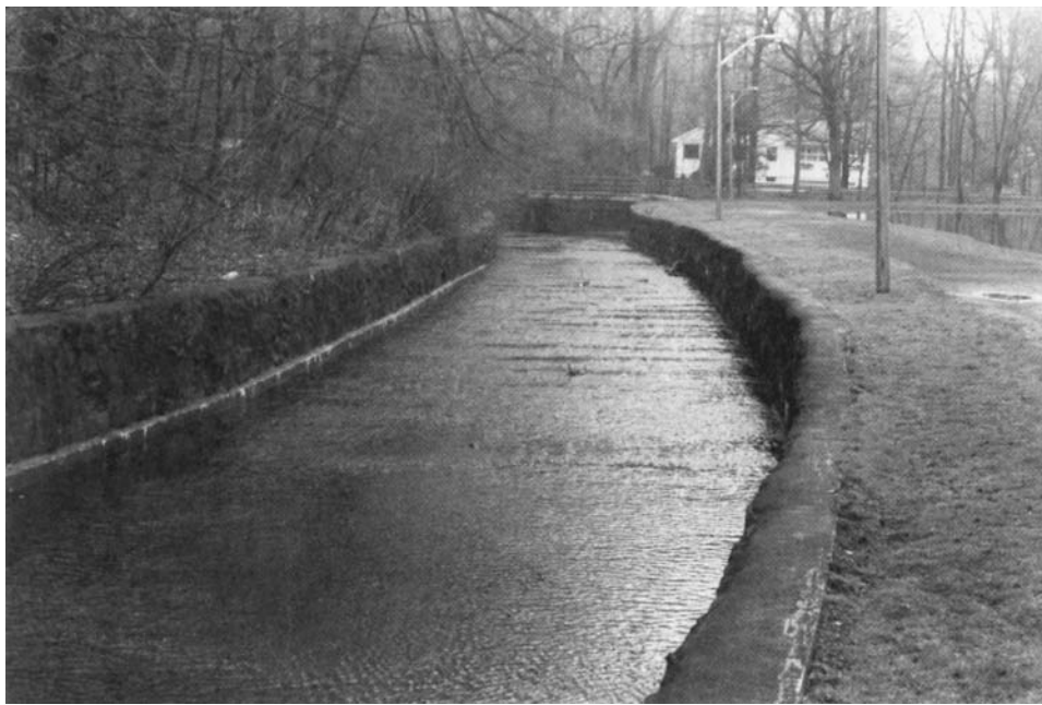
FIGURE 6-2 Open channels are often used to convey stream flow in developed areas. This channel has a rectangular shape with stone sides.
