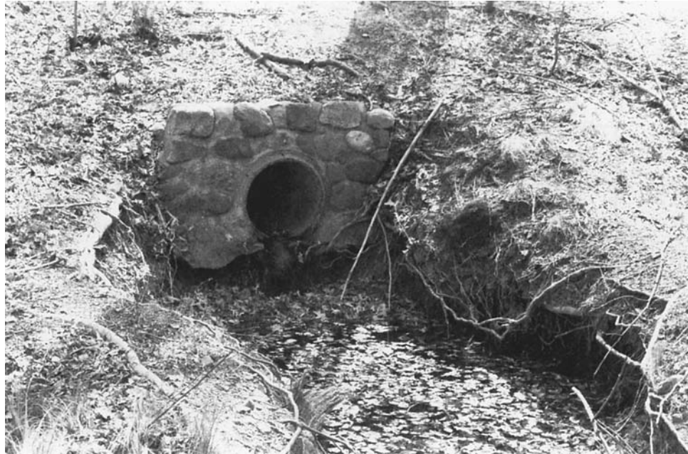
FIGURE 12-15 Storm sewer outfall with severely eroded ground immediately downstream.
