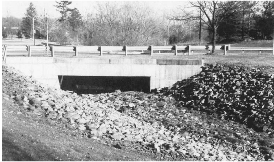
FIGURE 13-4 Extensive riprap protects the trapezoidal channel on the downstream side of this new concrete box culvert.
