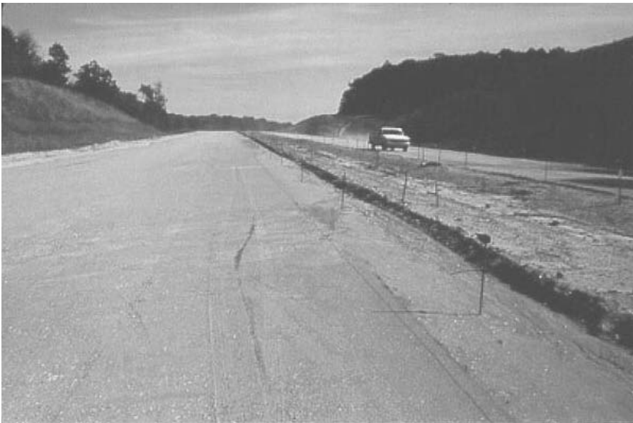
FIGURE 5.2 Compacted aggregate base before placing the hot-mix asphalt or portland cement concrete layer of a paved road.
