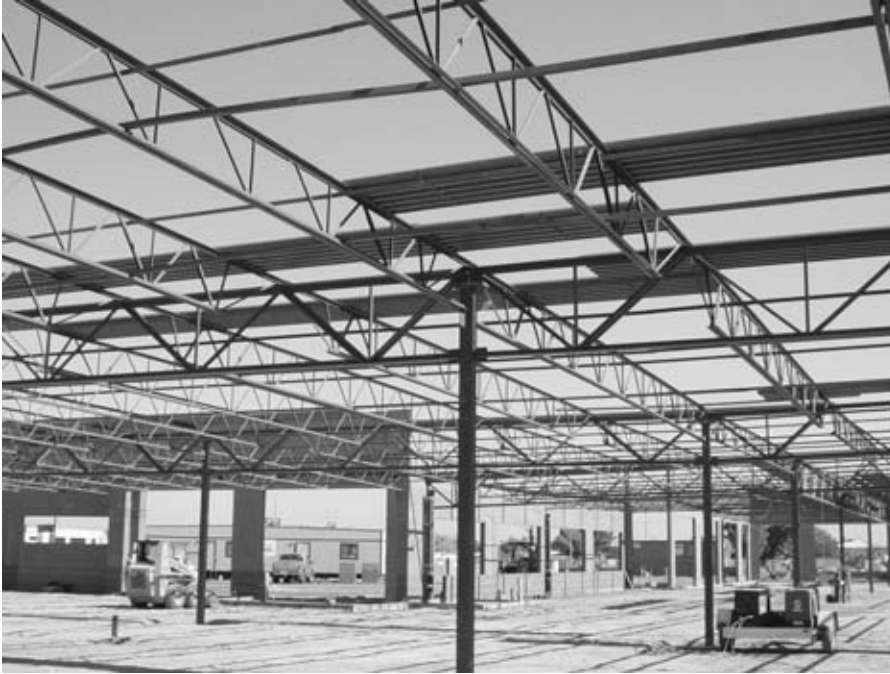
FIGURE 3.1 Truss made of structural steel for the structural support of a building.
