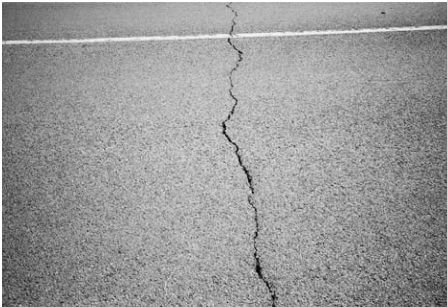
FIGURE 9.8 Thermal cracking resulting from the use of too stiff asphalt in a cold climate area.
