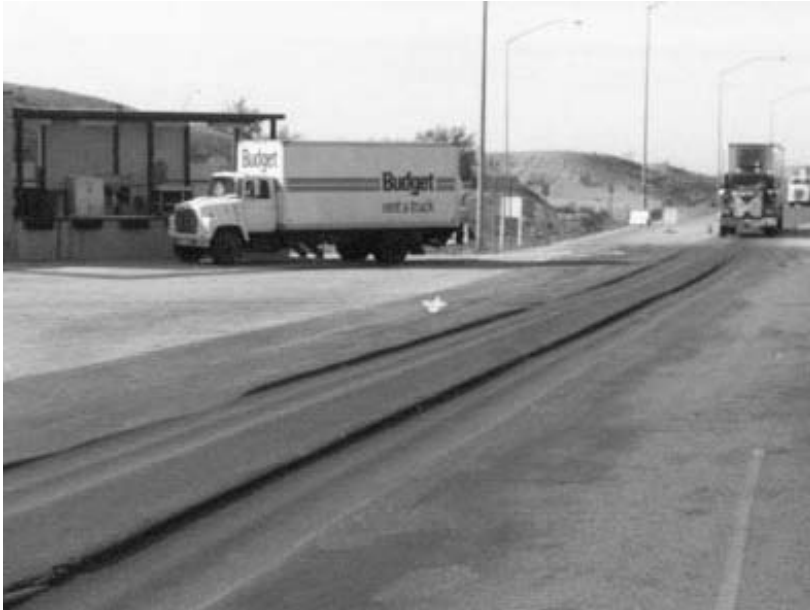
FIGURE 9.9 Rutting that could result from the use of too soft asphalt.
