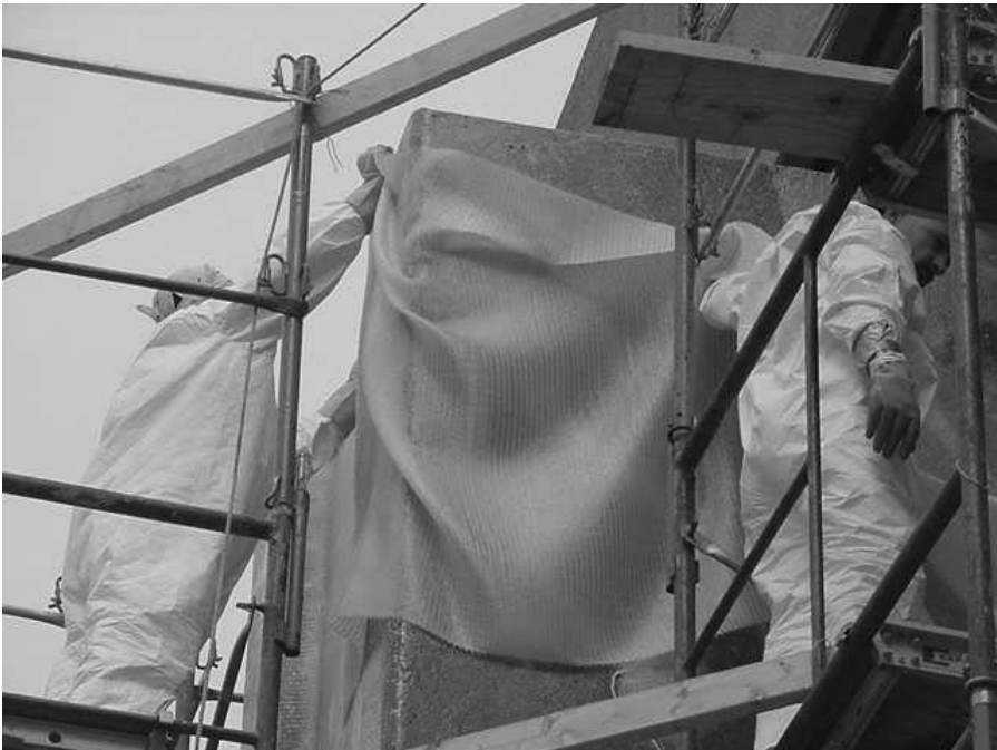
FIGURE 11.6 Wrapping an old structure with glass fiber-reinforced polymer (FRP) composite (Wabash Avenue pier, Baltimore, MD).
