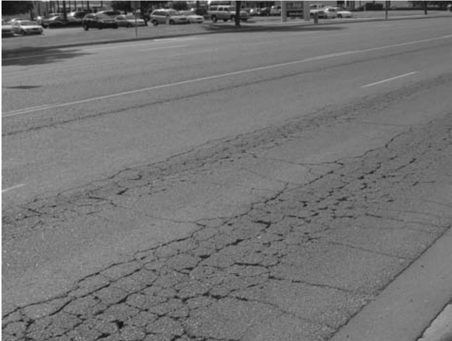
FIGURE 1.15 Fatigue failure of asphalt pavement due to repeated traffic loading.
