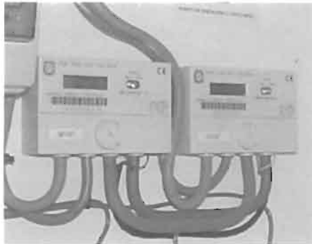
Figure 3 A pair of meters measuring import and export of electricity into a building and outputting pulse data to a monitoring system. (Photo EETS.)
