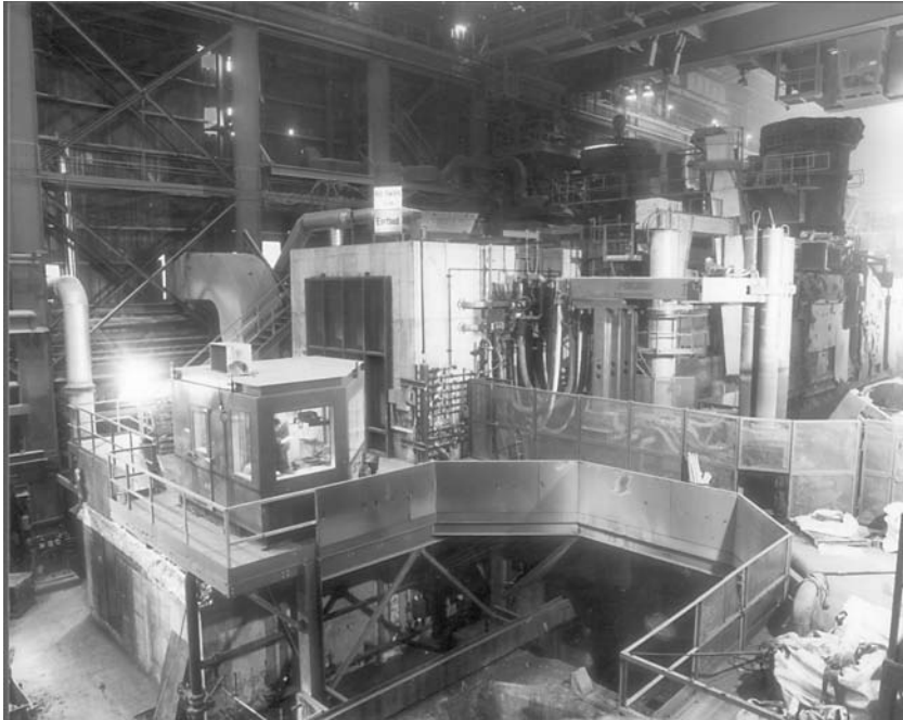
Figure 3.2 Ladle furnace at Sheerness Steel controlled by a PLC (Courtesy of Sheerness Steel)
