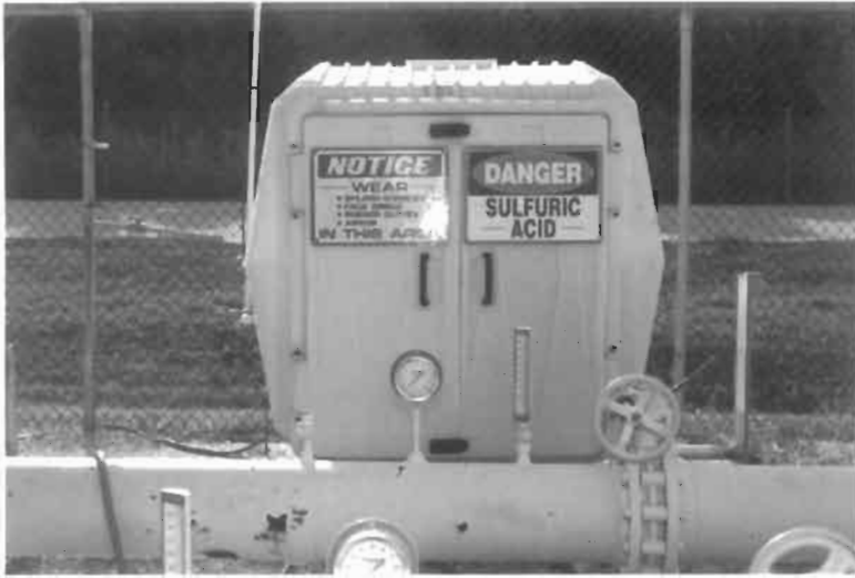
Figure 3.13 In-line addition of sulphuric acid to a recirculating cooling system in St. Petersburg, Florida
