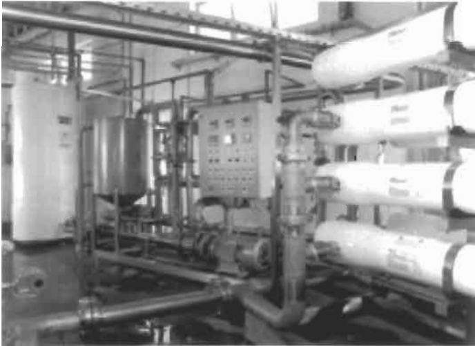
Figure 5.16 Reverse osmosis plant at Forsell and Sons Ltd
