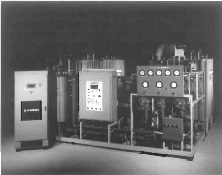
Figure 5.7 Ionics Aquamite XX EDR unit for Doswell combined cycle facility
