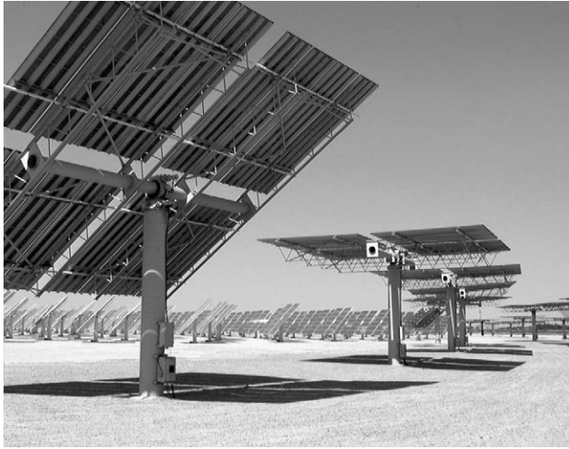
FIGURE 3.22 Detail of a heliostat.
