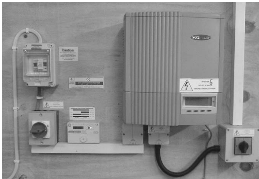
Figure 10-41 A typical inverter setup.
