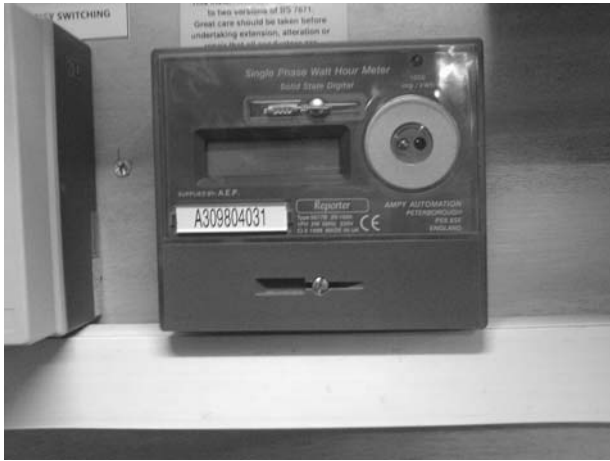
Figure 10-45 Watt hour meter.
