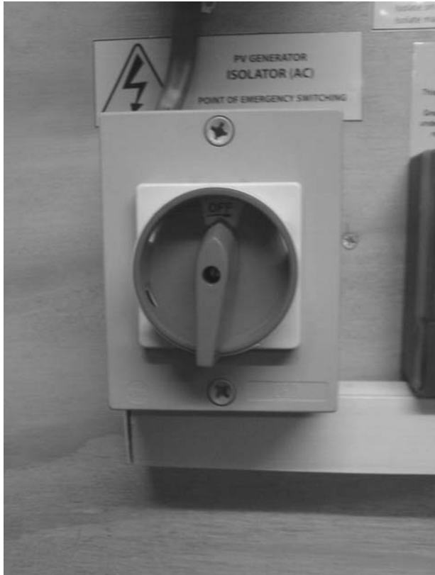
Figure 10-44 Solar DC isolator switch.
