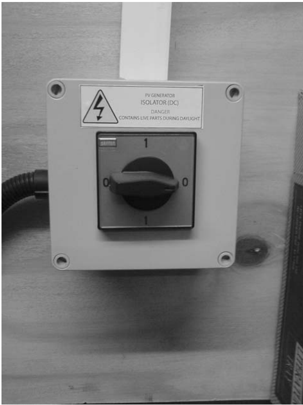
Figure 10-42 Mains isolator switch.
