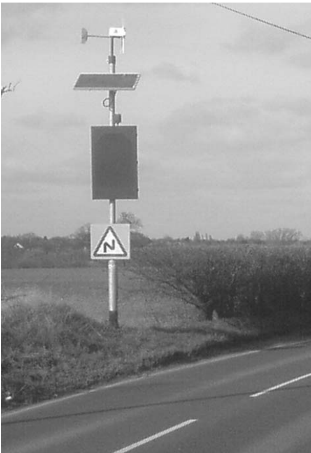
Figure 10-36 A road sign powered by renewable energy.
