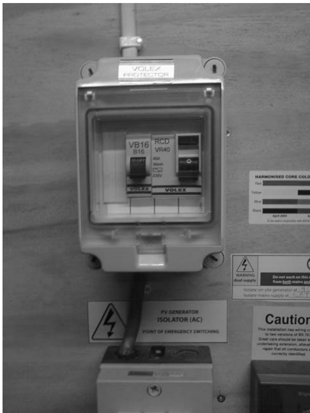
Figure 10-43 Mains circuit breaker.
