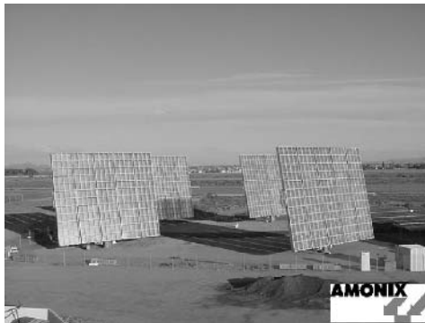
Figure 11.38 Amonix 100-kW high-concentration Fresnel lens array at the Glendale, California Airport
