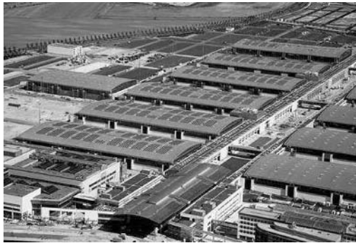
Figure 17.28 Central PV system installed on the roof of the new fair in Munich, Germany ( Source: Siemens Solar )
