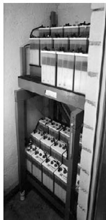
Figure 18.11 A battery in a photovoltaic system with a rated capacity of C_{10} = 37.5 Ah and a rated voltage of 168 V (flat-plate technology, 28 blocks of 6 V connected in series, Picture courtesy Fraunhofer ISE)
