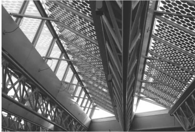
Figure 22.31 Atrium roof of the Brundtland Centre building from the inside. Because the saw-tooth roof casts a shadow on the modules, some of the cells are fake. This solution achieves a more elegant look from the inside. Reproduced with permission by BEAR Architekten T. Reijenga
