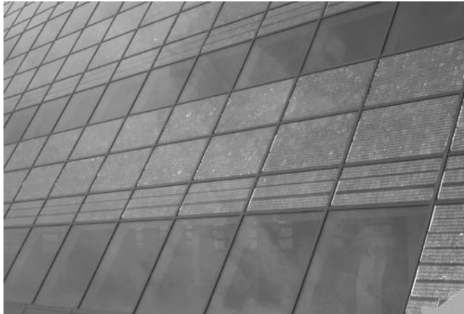
Figure 22.39 Schüco façade profile system in the Doxford building (UK). See also caption at Figures 22.4 and 22.18. Reproduced with permission by BEAR Architecten T. Reijenga
