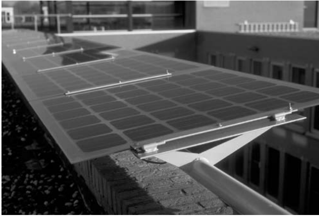
Figure 22.42 Canopy at the eaves of a roof. 6.2 kWp PV system at an office building in Gouda (NL). Reproduced with permission by BEAR Architecten T. Reijenga
