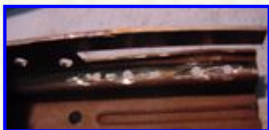
I ended up using a cut-off wheel on my Dremel tool to sever the last bits of weld. I do not recommend drilling the welds out as I did. Simply cut the welds out from the inside, using the edge of a fiber cut-off wheel. The holes that I left in the bracket made it so thin at some points that welding melted parts of the bracket.
