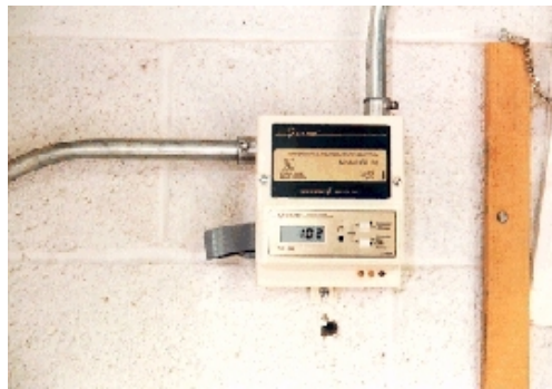
Figure G-8. Differential Temperature Controller
