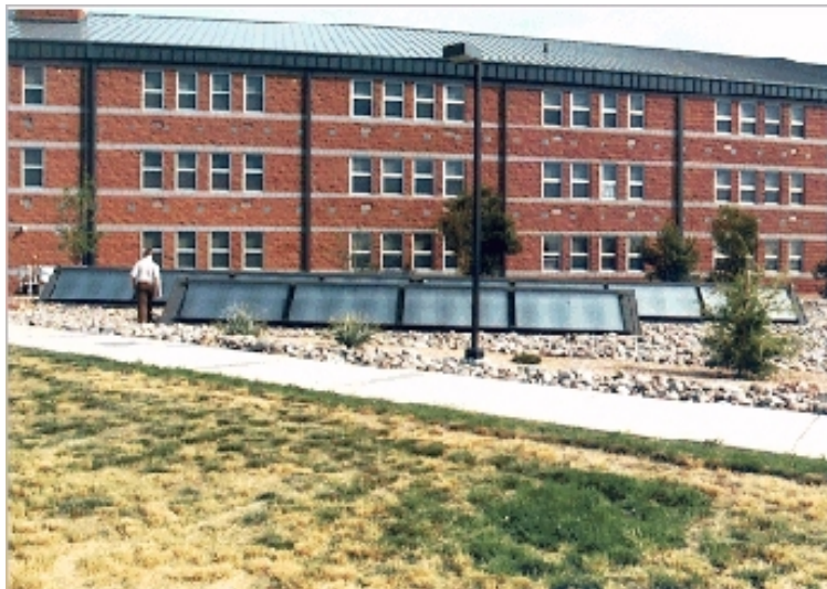
Figure G-1. Photo of Collector Arrays
