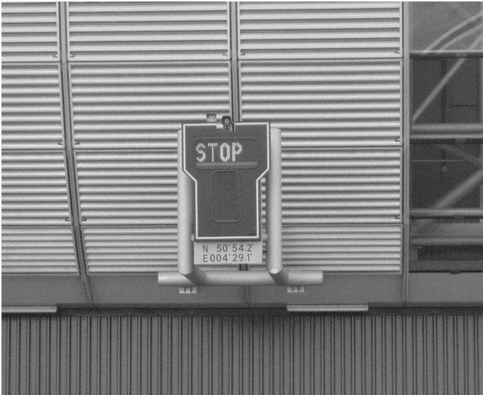
Figure 9-14 Honeywell's VDGS installation at Brussels airport (Photo: A. Kazda)
