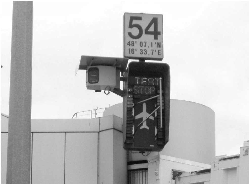
Figure 9-12 Typical installation of the Safegate guidance system (Photo: A. Kazda)
