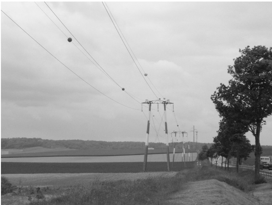
Figure 3-10 Marking high tension transmission lines (Photo A. Kazda)
