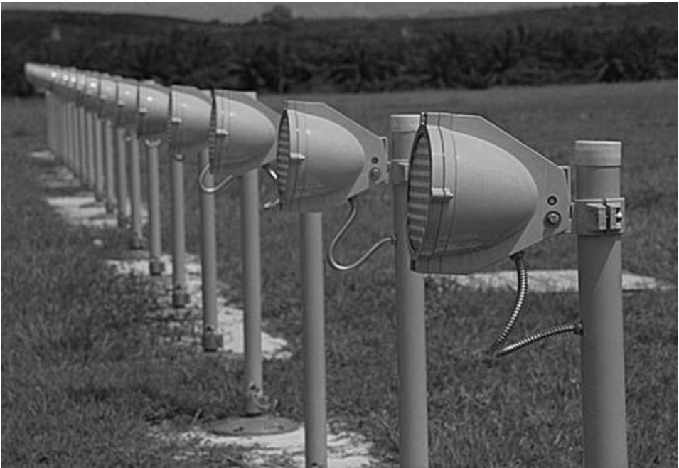
Figure 15-16 Honeywell High Intensity Approach Light Type ATR 12 (Photo: Courtesy Honeywell Airport Systems)
