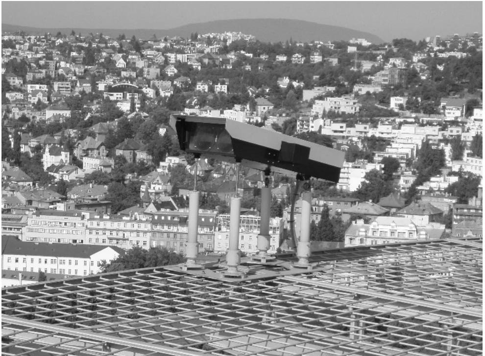
Figure 15-21 Typical HAPI installation at elevated heliport, (Photo: A. Kazda)
