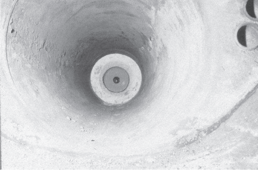
Figure 4-6. Combustion Chamber and Fire Tubes. Two-pass Boiler
