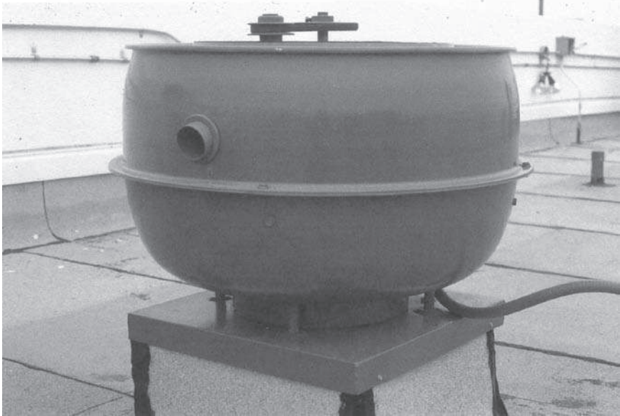
Figure 8-2. Power roof ventilator
