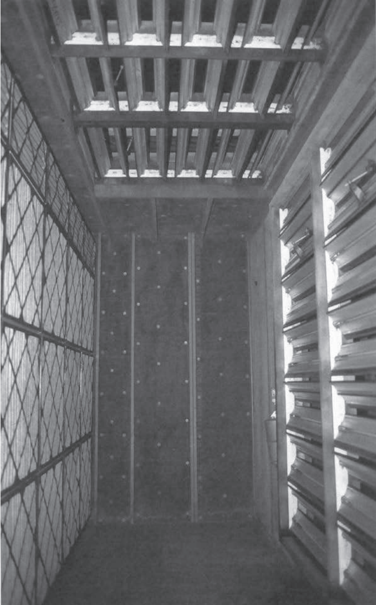
Figure 9-13. Opposed blade dampers in mixed air plenum. Notice blade action for opposed blade and parallel blade dampers.
