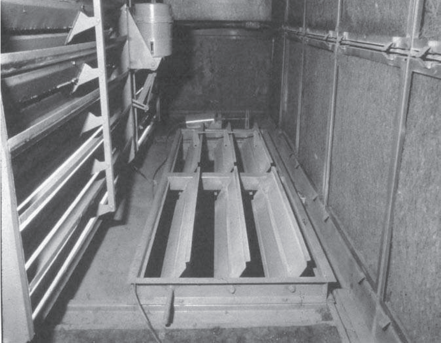
Figure 9-14. Parallel blade dampers in mixed air plenum. Notice blade action for opposed blade and parallel blade dampers.
