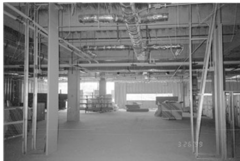
Figure 3.11 Ductwork system with several area changes.
