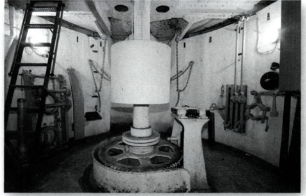
The lower chamber of the 10cm gun turret of Feste Wagner. The counterweight in the centre of the column eased the raising and lowering of the gun in the chamber above. The wheel at the bottom of the column raised the entire turret off its forward armour collar. (Dan McKenzie)
