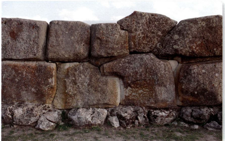
A defensive wall near the Sphinx Gate of Alacahöyük. A perfect example of cyclopean polygonal masonry laid without any mortar. The stone blocks fit in so well that a sheet of paper could not be shoved in between them; the two blocks in the centre have been given a special projection and hollow to make them fit better.
