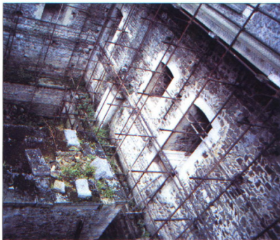
The blind basement and the first floor of the donjon at Falaise.
