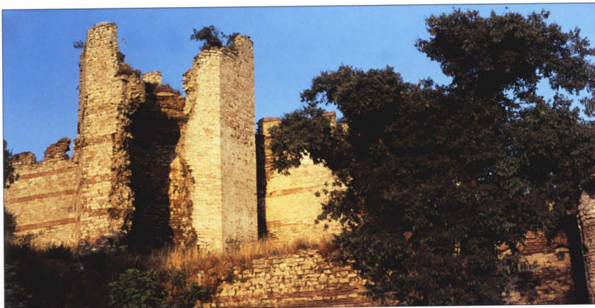
A very damaged octagonal tower from the inner section of the Theodosian walls, located just to the south of the Golden Gate.
