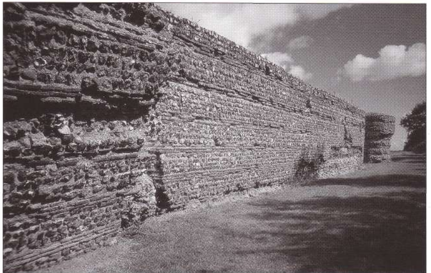
South wall of Burgh Castle-Gariannum, part standing, part toppling, part fallen. The standing section retains all its facing-flints, separated by rows of brick bonding courses, 3.2m thick at base and 4.5m high – probably its original height except for a parapet. (Author's collection)
