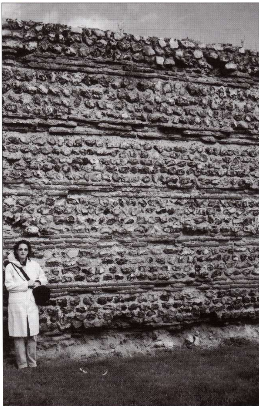
South wall of Burgh Castle- Gariannum , a close-up view showing the construction. Brick bonding courses usually provided horizontal stability by running from the facing into the centre of the core. However, here at Burgh Castle they are only surface deep. (Author's collection)
