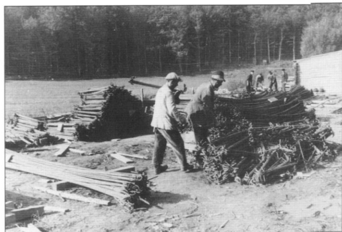
TOP The shuttering wood, squared timber, planks and round timber used in the construction of the West Wall in the period to 28 November 1938 (both Army and Luftwaffe).
