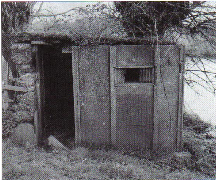
A fate that has befallen many pillboxes: a collapsing 'Stent' prefabricated pillbox at Eckington Bridge, Worcestershire. The spaces between the panels were filled with a weak concrete mix. The foundations of the pillbox are being undermined by the River Avon, which in 1940 was one of the Midland stop-lines. (MW)
