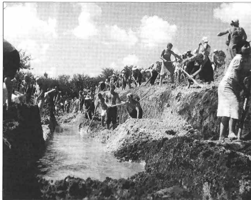
Impressed civilian labourers dig an anti-tank ditch. Hundreds of thousands were employed in such tasks and were instrumental to the defence of the Motherland. They turned out for work regardless of age, sex, or physical condition. The clothing and footwear of the women here are clearly inadequate for this type of work. (CMAF)
