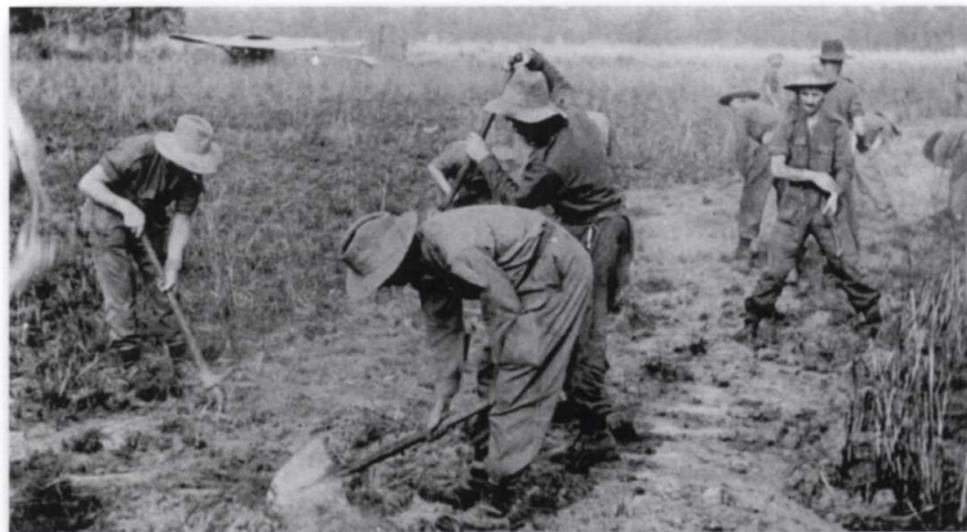
Chindits hard at work flattening an area of dry paddy for a light-plane airstrip. (SE 7956)
