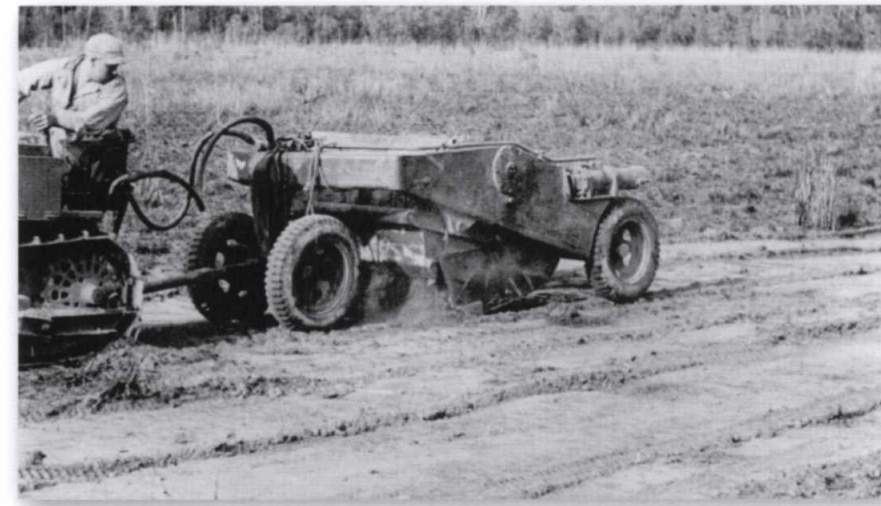
A US Army engineer uses a grader, landed by glider, to level an airstrip in Burma to make it suitable for transport aircraft. (SE 7932)
