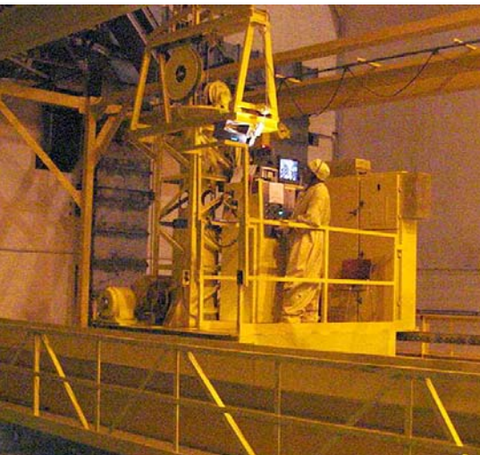
Main fuel handling bridge during 13RFO and before the modification
