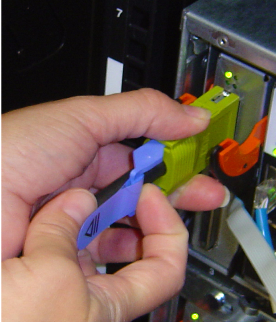
Figure 2-1: Connecting InfiniBand Cables
